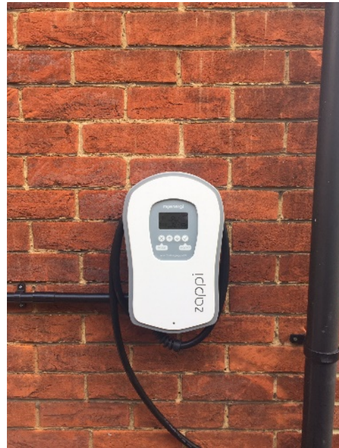
Figure 9: A wall-mounted EV chargepoint 16
