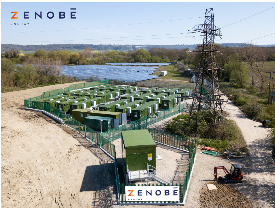
Figure 3: Zenobe's 29 MW battery storage site at Aylesford in Kent, co-located with a solar farm 8
