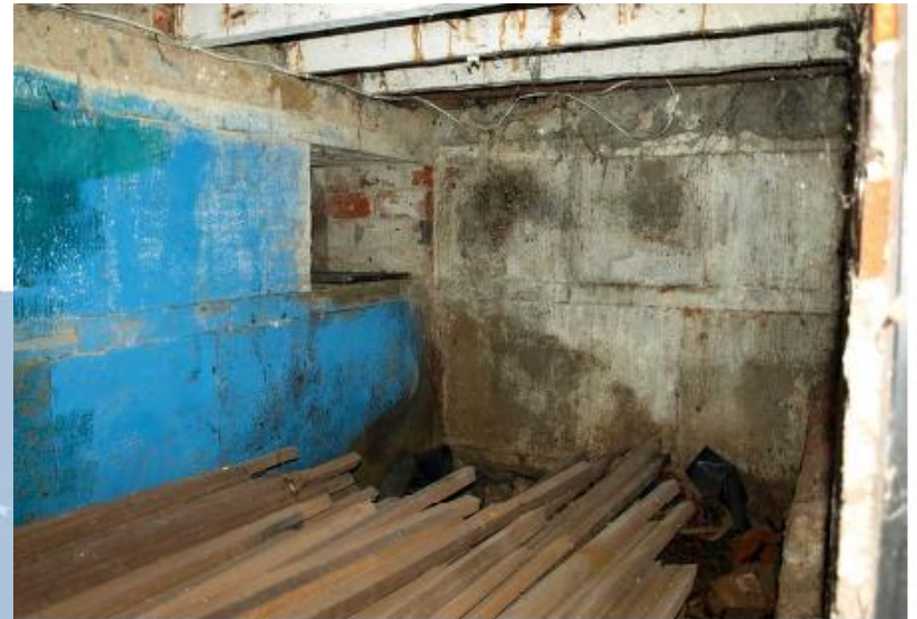
The historic baths below the suspended ground floor are currently used for storage
