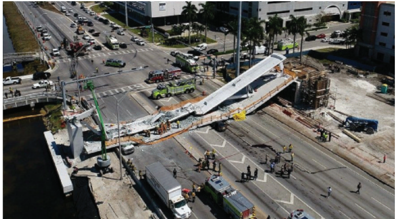
Picture of the collapsed Florida International University bridge.
